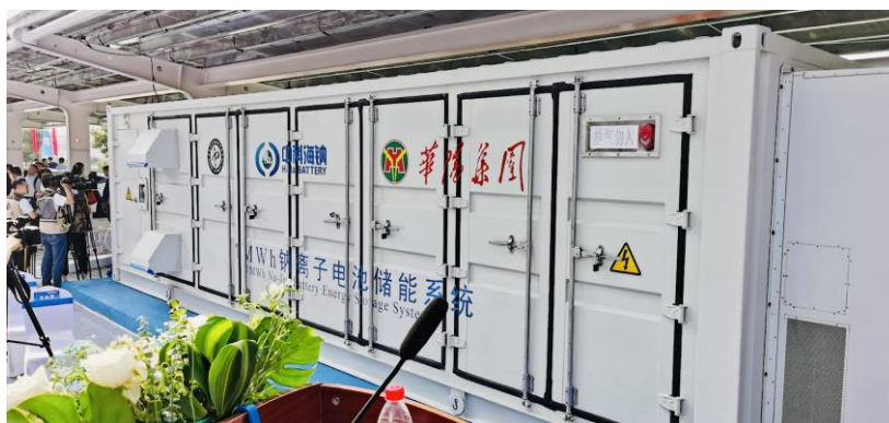
Figure 39: A 1 MWh SIB-based energy storage system put into operation by HiNa Battery Technology Co., Ltd.. Reprinted with the permission from 335 , Copyright HiNa Battery Technology Co., Ltd.
