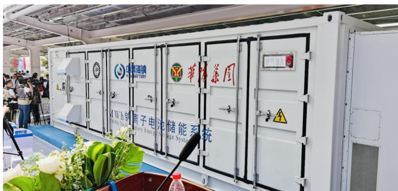
Figure 39: A 1 MWh SIB-based energy storage system put into operation by HiNa Battery Technology Co., Ltd.. Reprinted with the permission from 335 , Copyright HiNa Battery Technology Co., Ltd.
