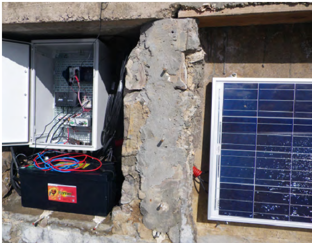
FIGURE 7. Photograph of the electrical setup embedded in the seawall.
